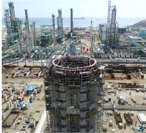
RAFFINERIE PETROPERU | Talara, Peru Komplettsysteme KCVC
